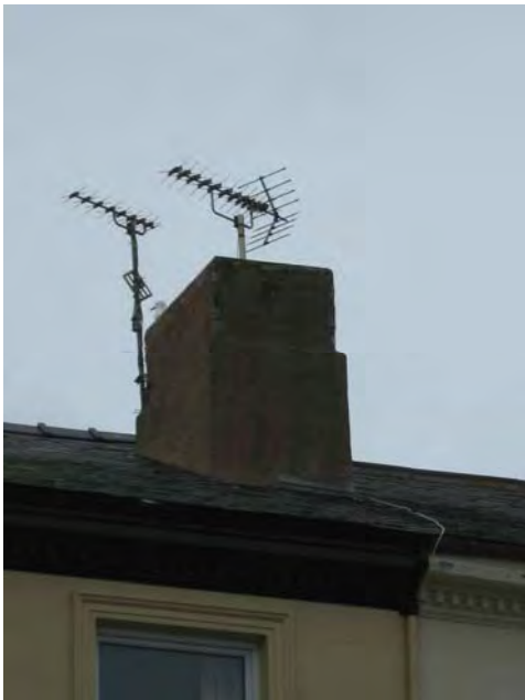
Aerials mounted on chimney stack
