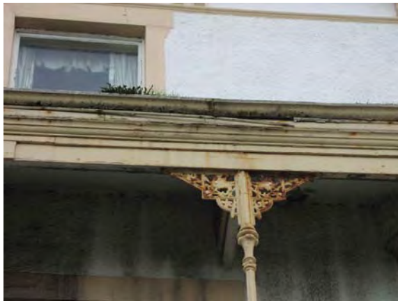
External iron work in need of maintenance
